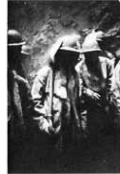
58. Shaft sinking: during 'blowing over' of shaft-bottom. President Steyn No.4, Welkom. 1969 (E9016)
